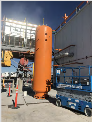
Johnstown, NY: Air Cooled Condensers
